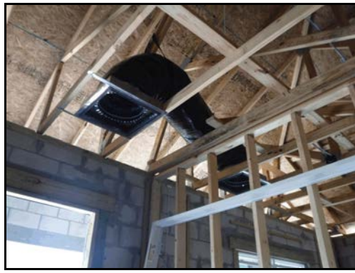
20. Master HVAC return vent not as per plan
