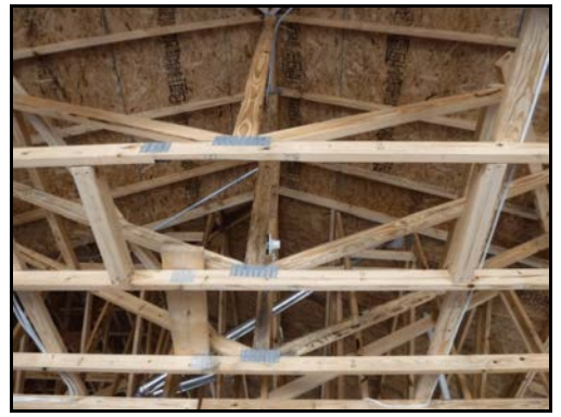
12. Plans call for receptacle above attic access in garage
