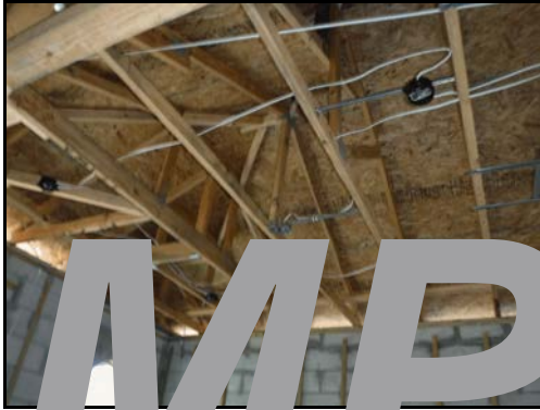
14. For lights needed to be installed, family room, bedroom, pendants in kitchen.
