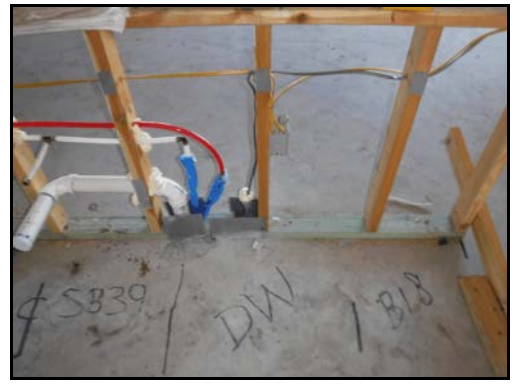
21. No power observed for dishwasher
