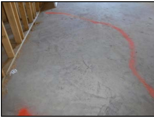
19. Large area of raised concrete in den, hall and family rooming
