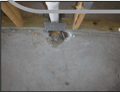
16. Void in concrete floor of laundry room and rear bedroom.
