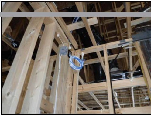
17. Low voltage wires in #4 bedroom.
