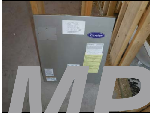
23. Carrier handler cabinet. Carrier handler cabinet.
