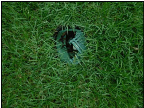
7. Damage to drain cover in right yard.
