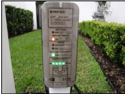
8. "Low salt" reading at pool equipment.
