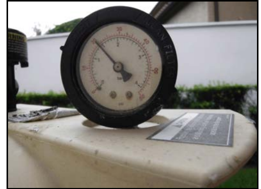
6. Pressure gauge at pool filter did not appear to function.
