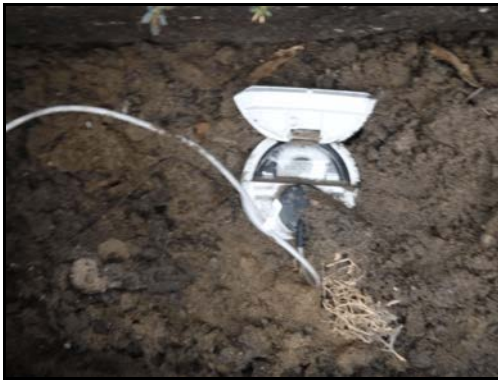
1. Movement at water meter leak detector.
