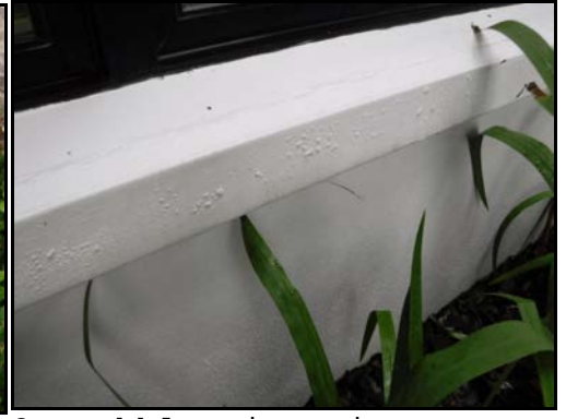
3. Bubbles in paint at office window sill.
