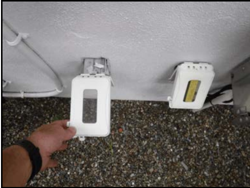
4. Electrical box on right side of house not secure in wall.
