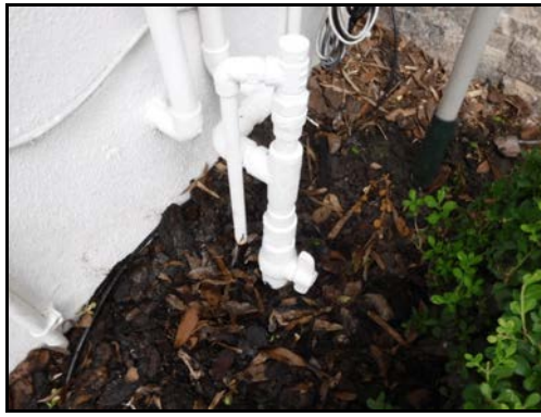
2. Meter movement maybe water leaking from pressure relief valve at main water shut off.
