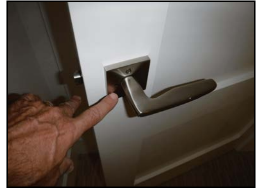
9. Missing lock pin in right guest bedroom door.
