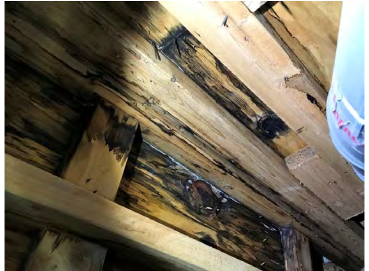
8. Stains on master bedroom wall maybe from previous roof leak associated with fireplace chimney.
