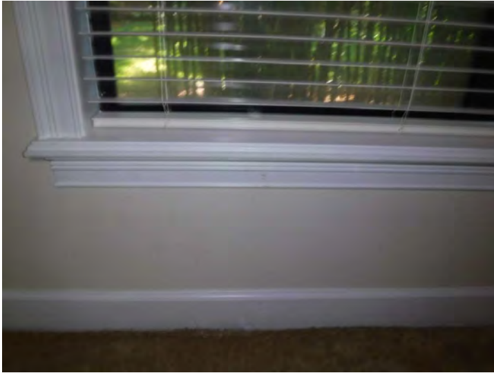
5. Possible previous water intrusion at the second bedroom on first floor.
