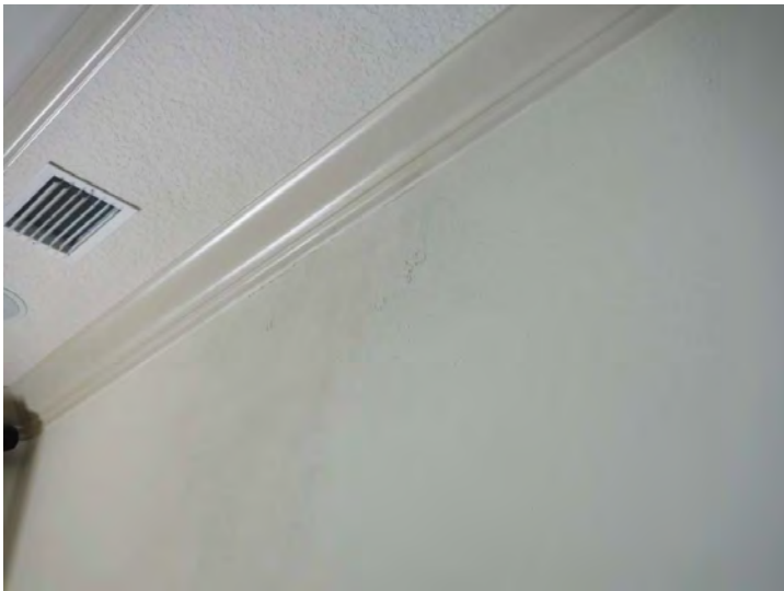
7. Blemishes on the drywall of the master bedroom.
