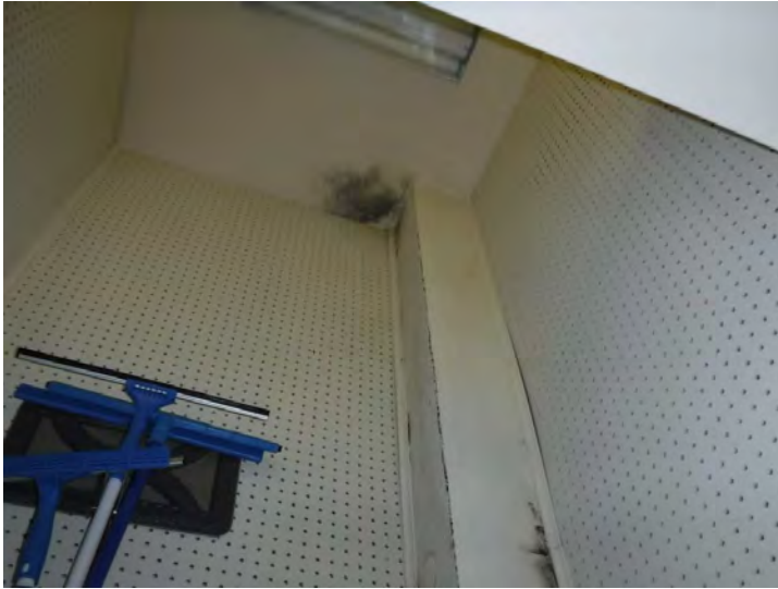
1. Mold in the corner of the pool / lanai storage closet.
