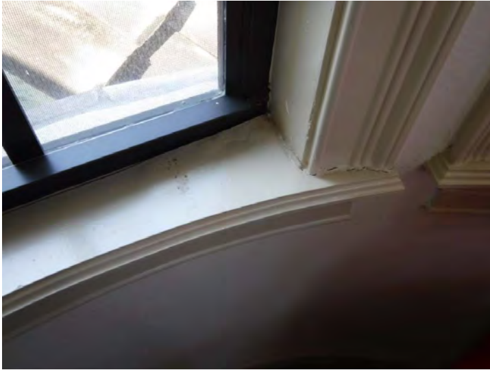
9. Water stains evident on the window sill of front right bedroom on the second floor
