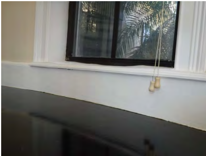
3. Damaged window sill and jamb at staircase.
