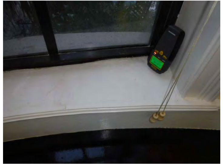
4. Elevated moisture in the window sill in the guest bedroom.
