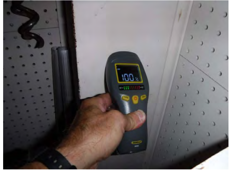
2. Elevated moisture in the corner of closet.
