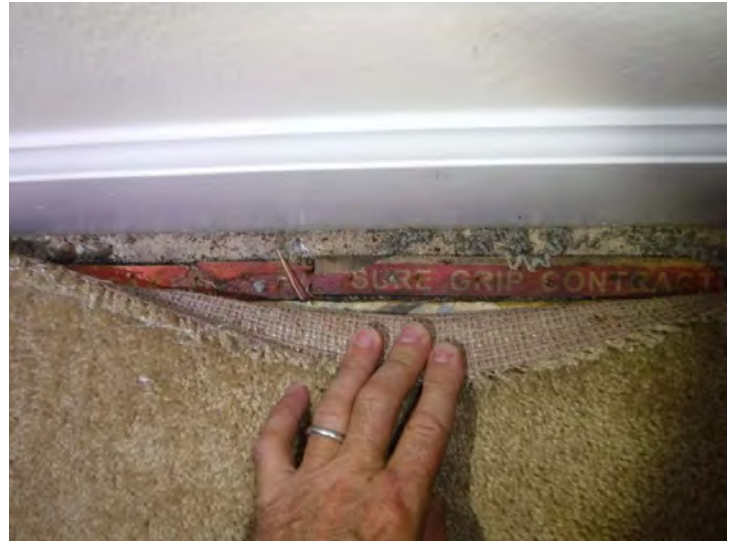
6 A little staining on the carpet tack strip of this bedroom, under window
